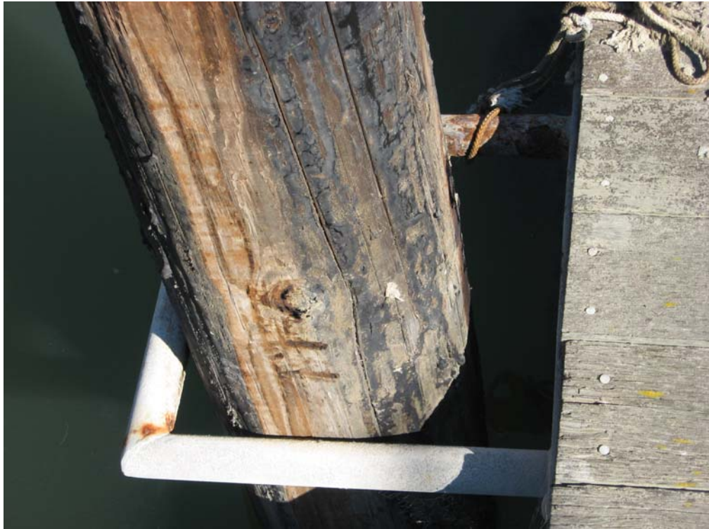
Guest Dock – Timber pile needing wrapping and new pile guide with rollers
