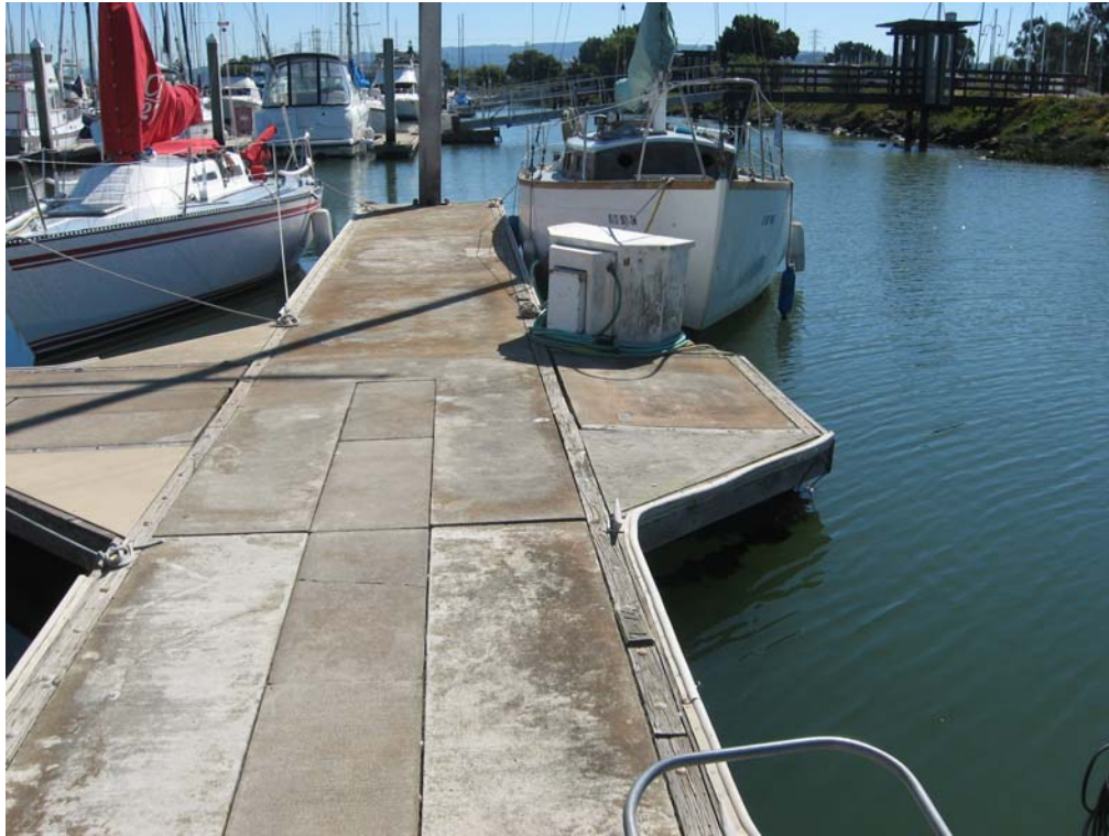
Dock 27 – Deteriorated dock surfaces
