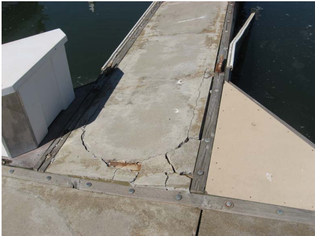
Dock 29 – Deterioration and damage
