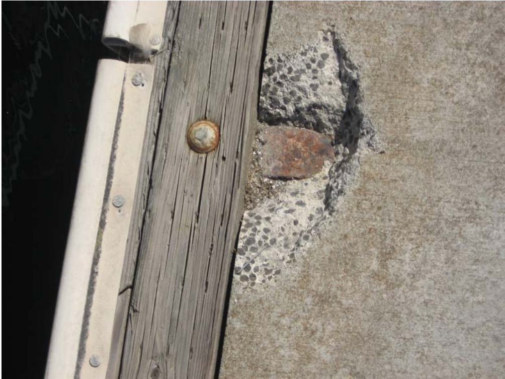
Dock 27 – Deteriorated concrete finger float
