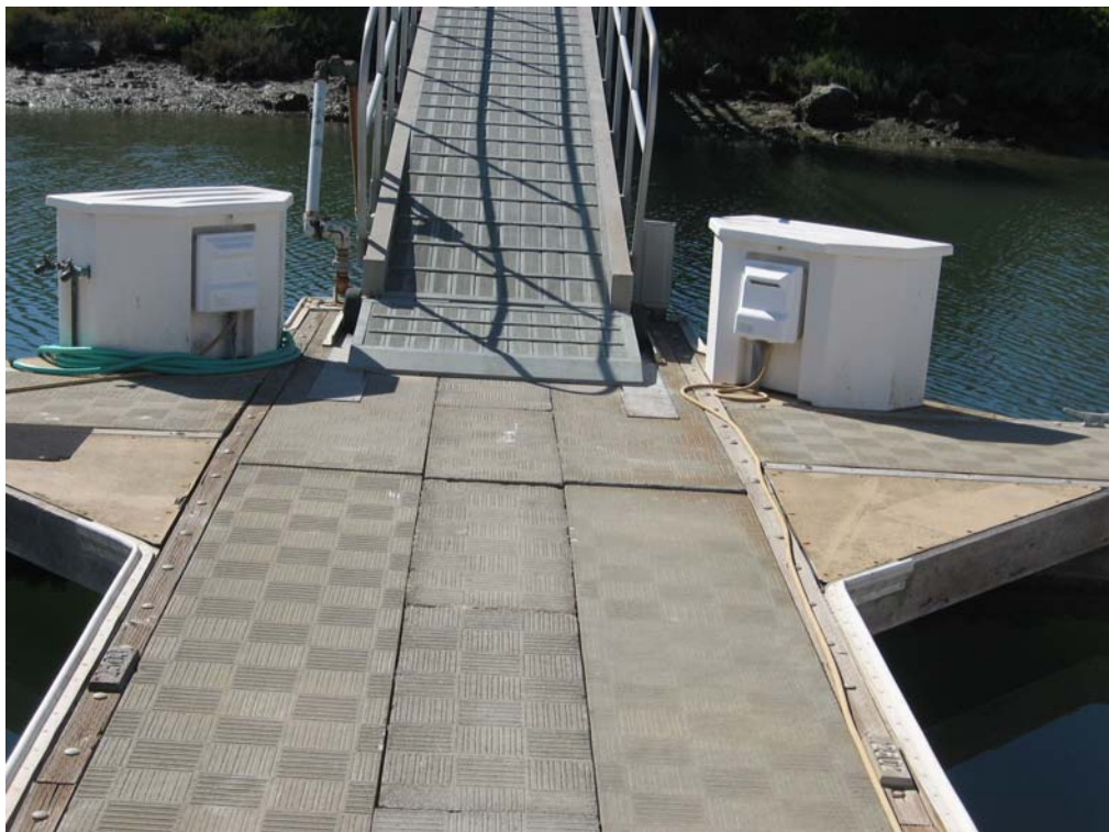
Dock 25 – Gaps in decking
