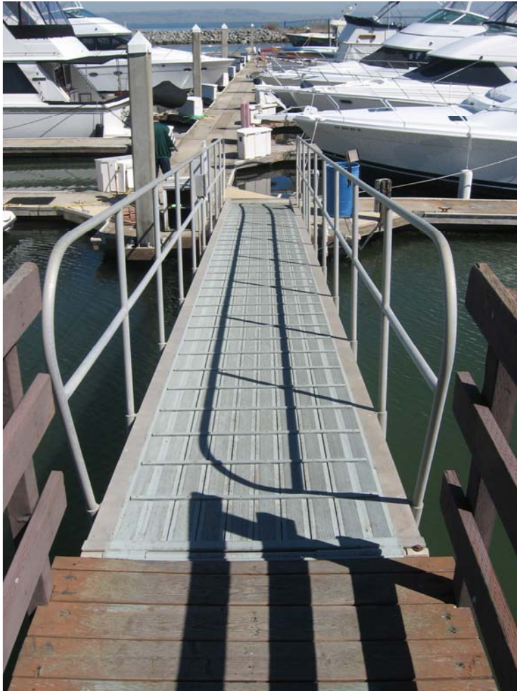
Typical old style gangway, sturdy but railing not meeting current codes
