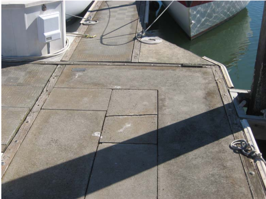
Dock 22 – Broken deck and gaps
