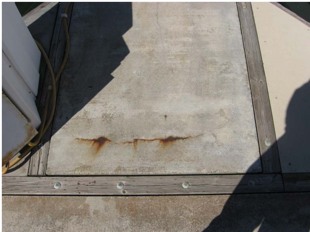
Dock 26 – Deteriorated concrete finger float
