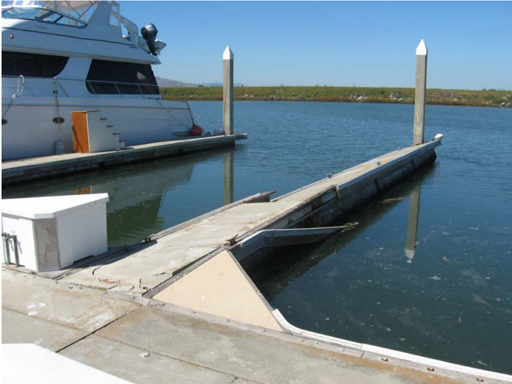
Dock 29 – Deterioration and damage
