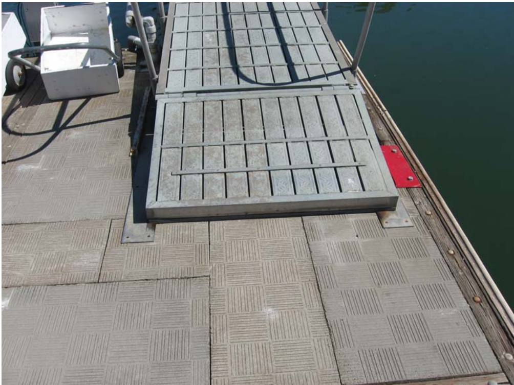
Dock 12 – Non-standard gangway toe plate
