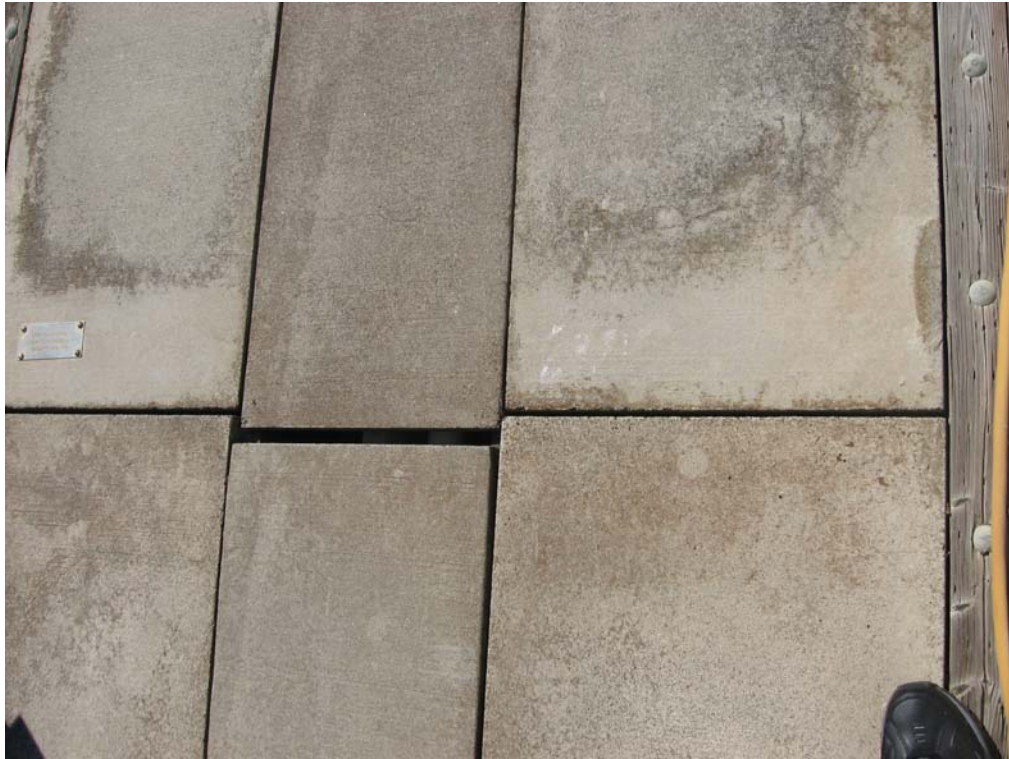
Dock 26 – Gaps in decking
