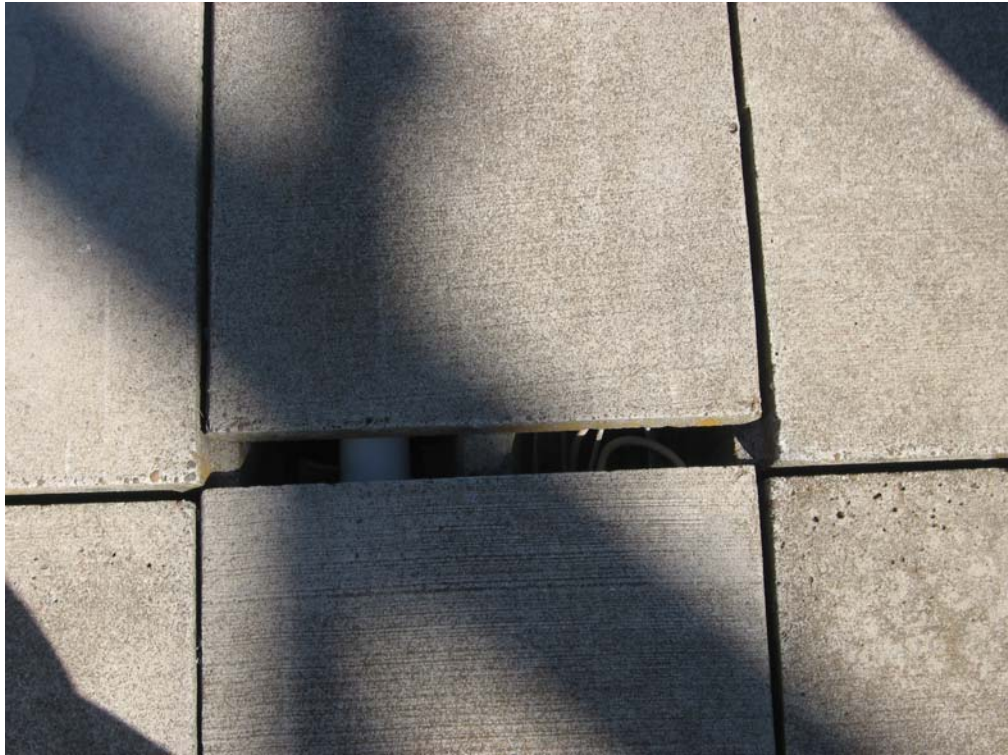
Dock 26 – Gaps in decking
