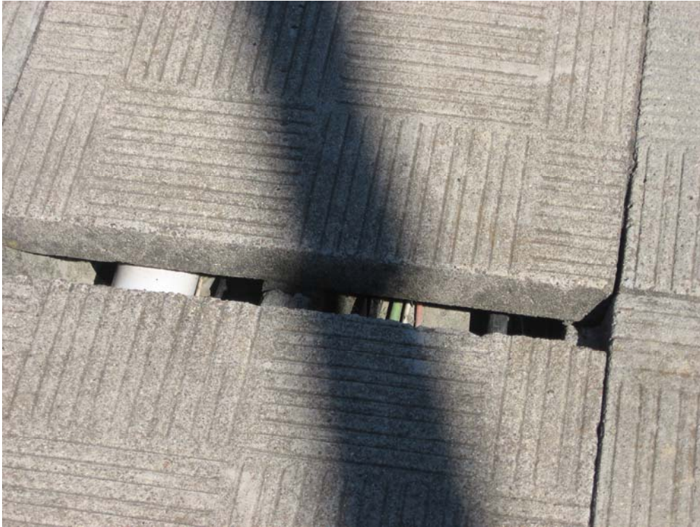
Dock 11 – Deck gaps
