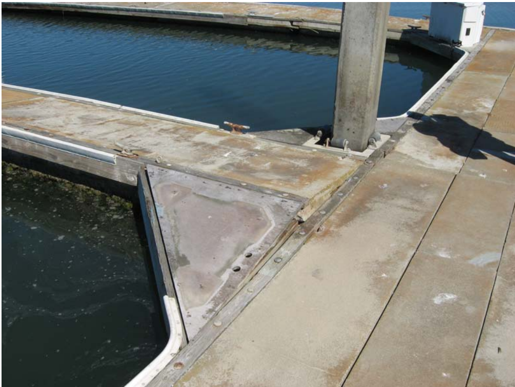
Dock 29 – Deteriorated concrete finger float
