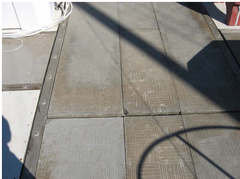
Dock 22 – Gaps in decking
