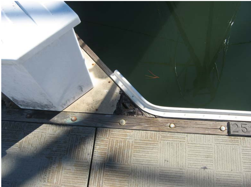
Dock 25 – Deteriorated knee brace plywood
