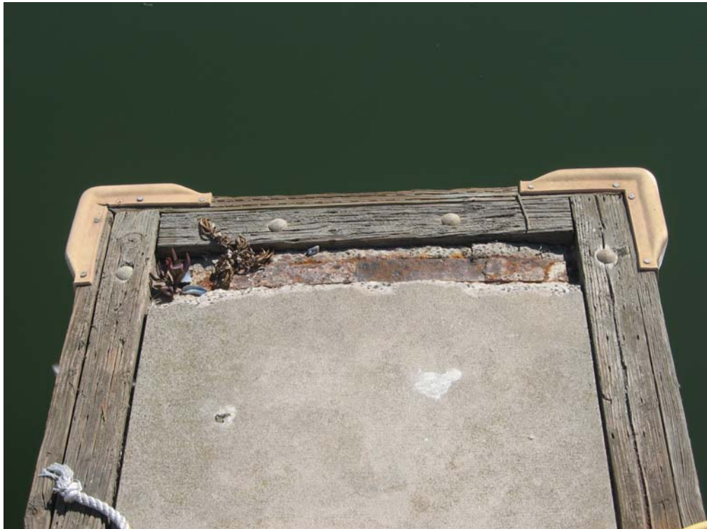
Dock 77 – Deteriorated concrete finger float
