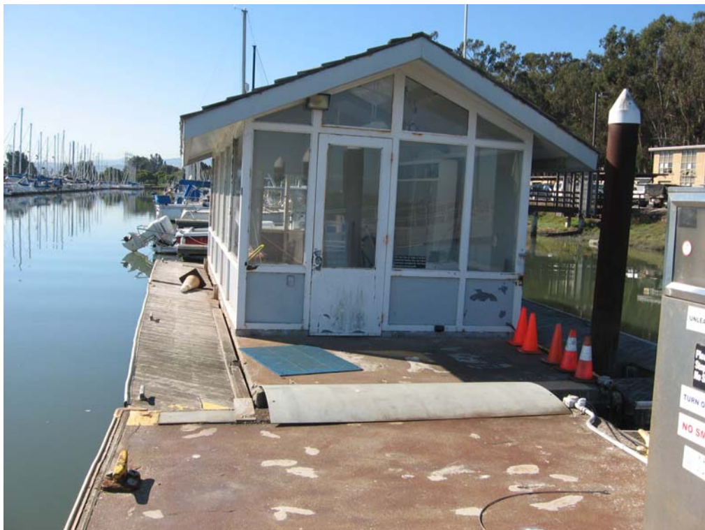
Fuel Dock – Unstable wood dock at utility building
