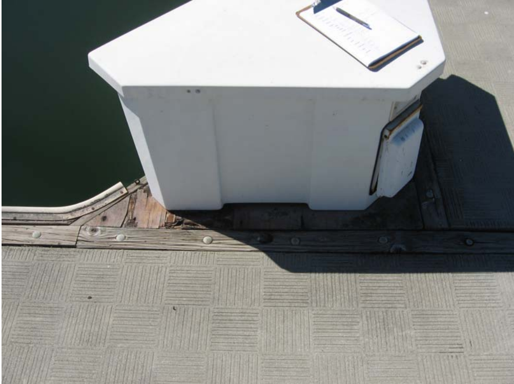
Dock 13 – Deteriorated knee brace plywood decking
